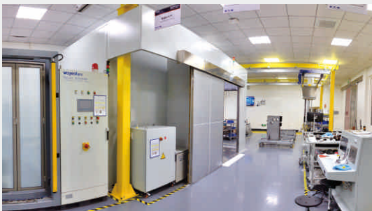
GSN gas tank assembly line
